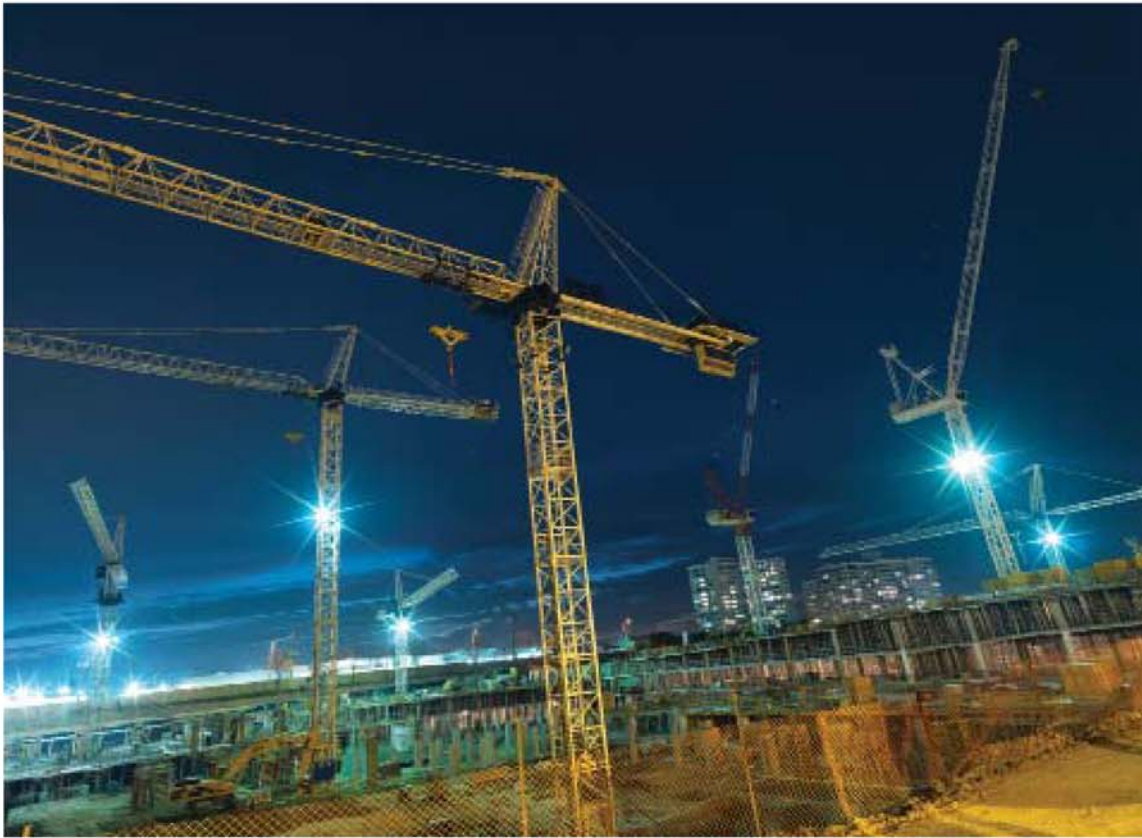
Eight cranes are working hard to build the components of World on Yonge in Thornhill.
